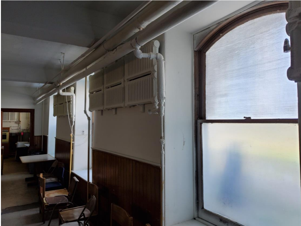
Typical Window Components covered in lead based paint on the date of the inspection
