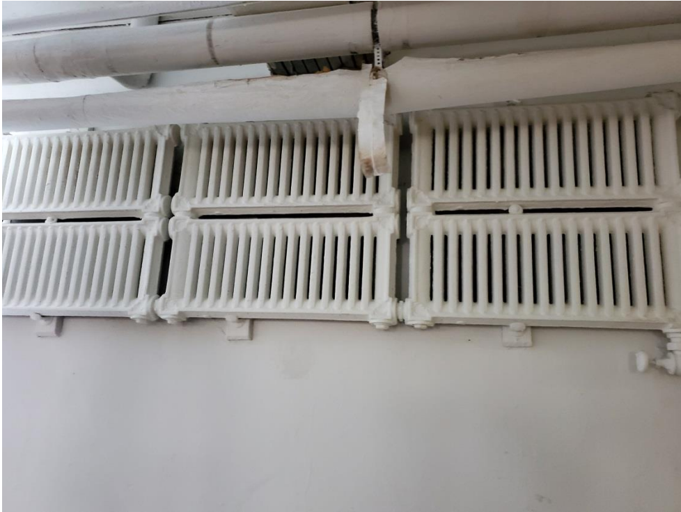
Typical Radiator covered in lead based paint on the date of the inspection
