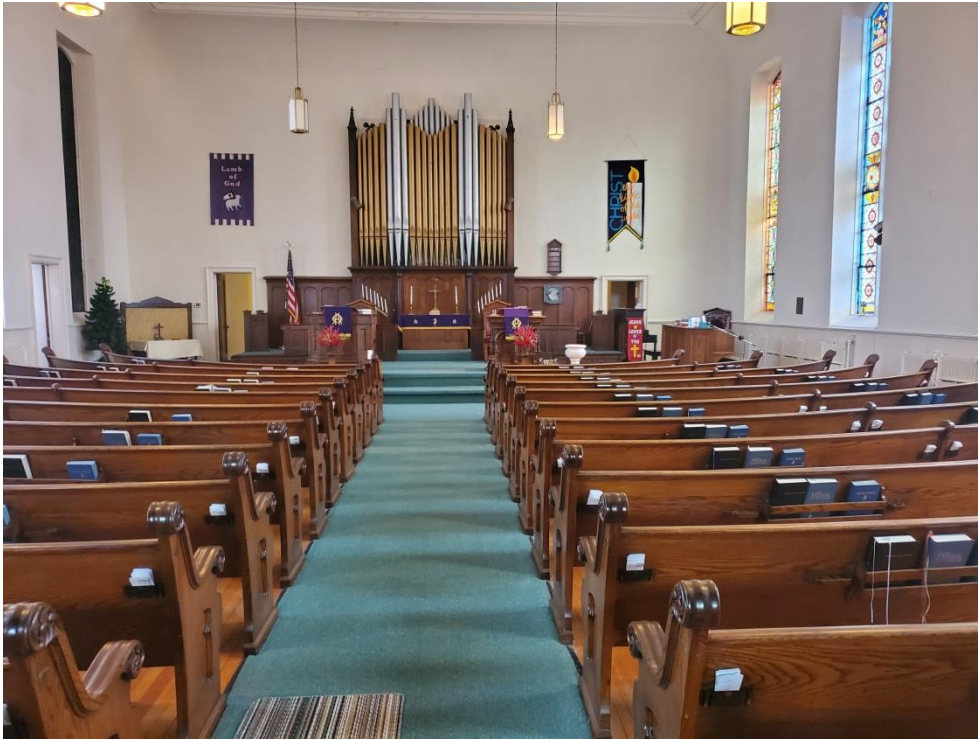
Typical Walls covered in lead based paint on the date of the inspection
