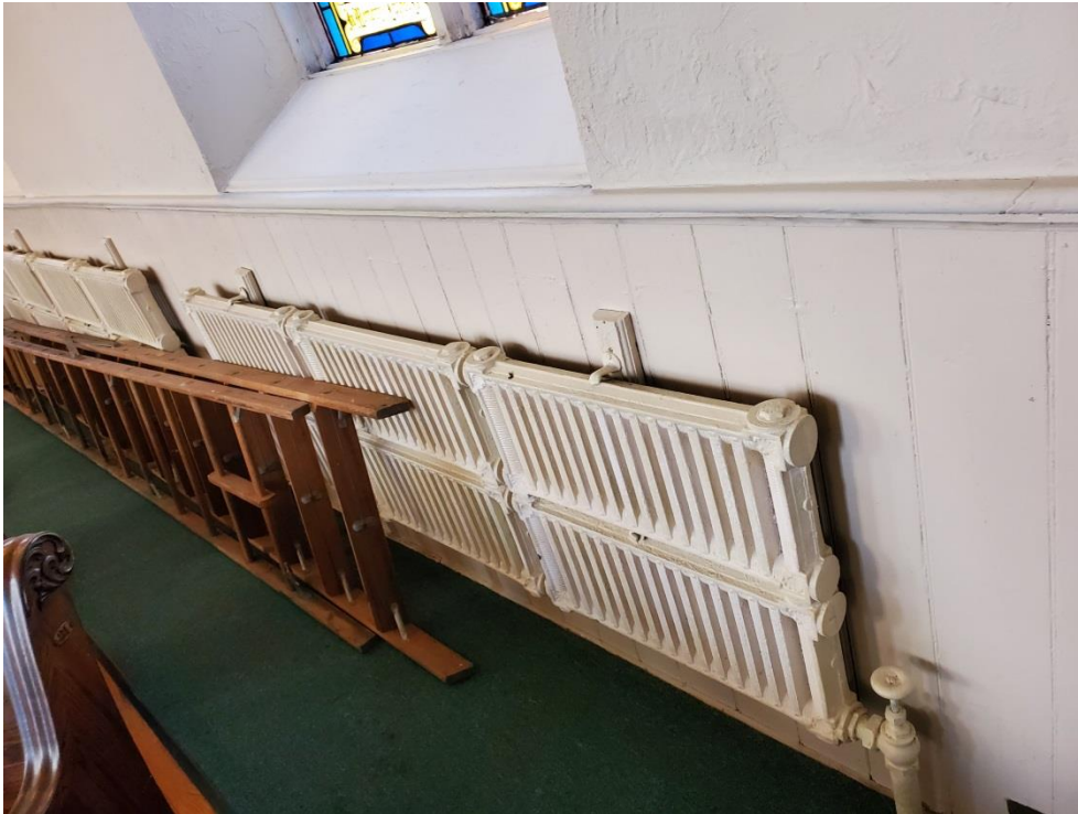
Typical Wainscoting and Radiator covered in lead based paint on the date of the inspection
