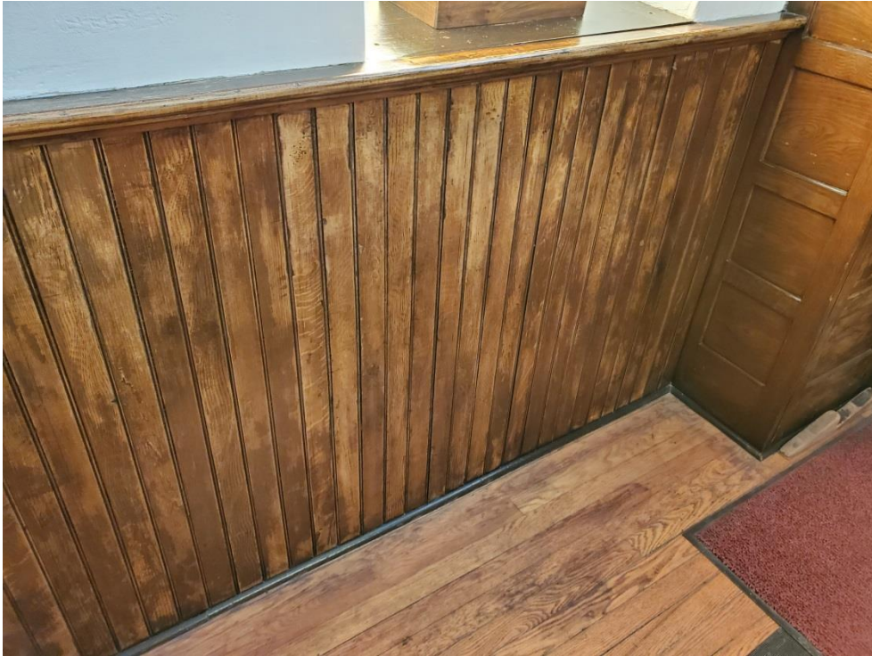
Typical Vanish Wainscoting covered in lead based paint on the date of the inspection
