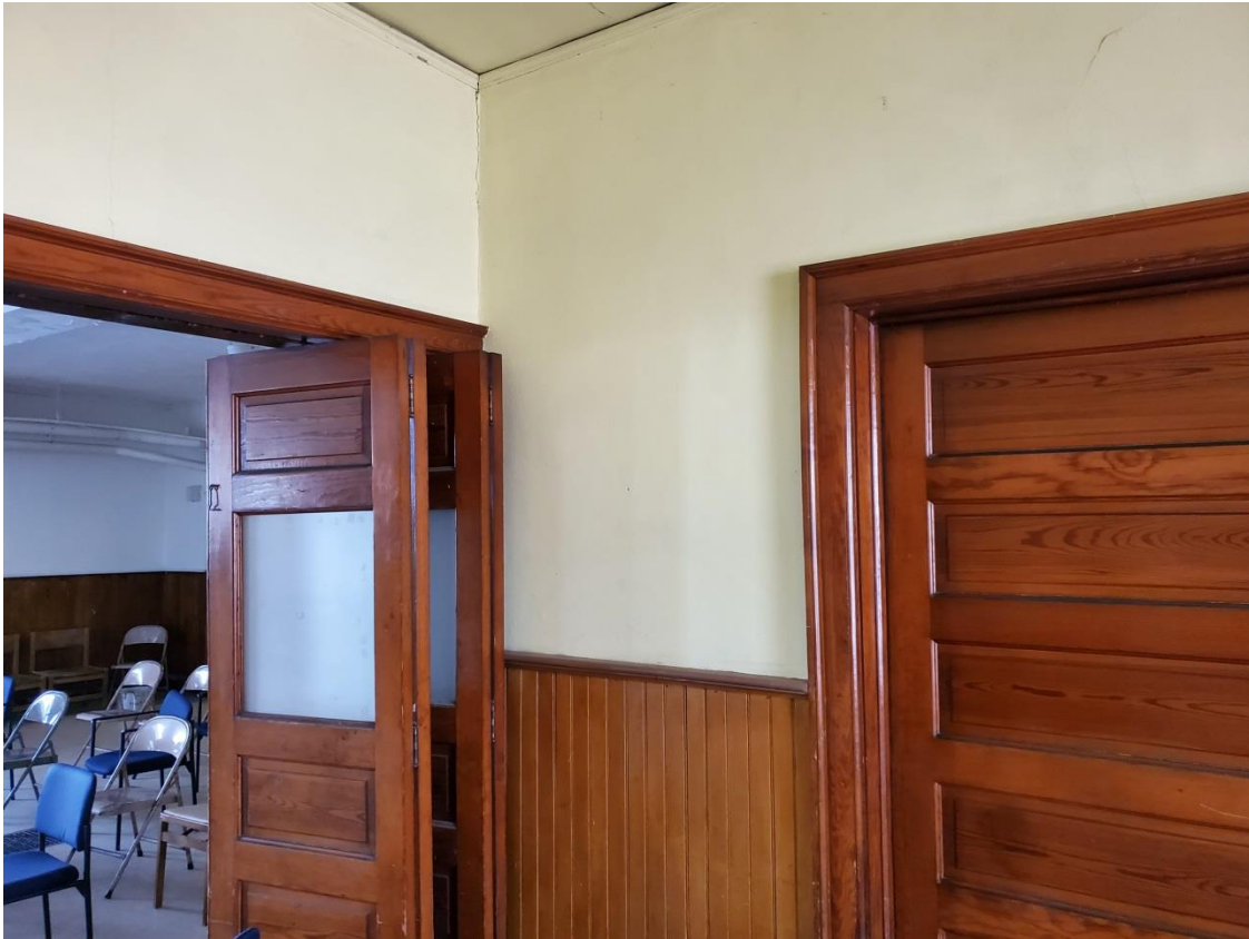
Typical Door Components covered in lead based paint on the date of the inspection
